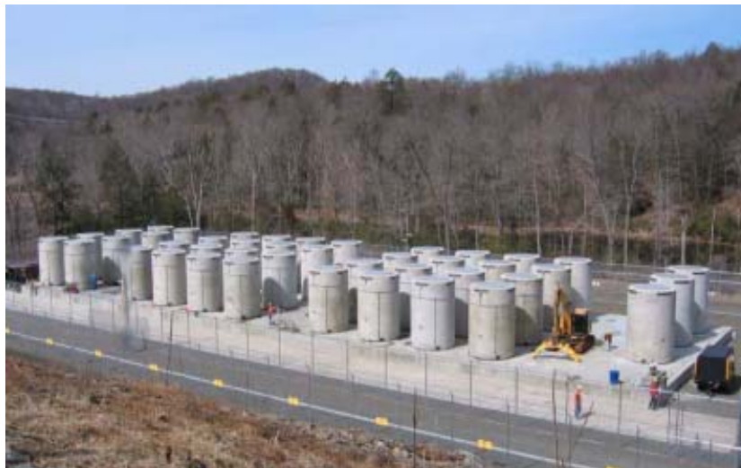
NAC installed HLW Canisters at Maine Yankee Project Site
